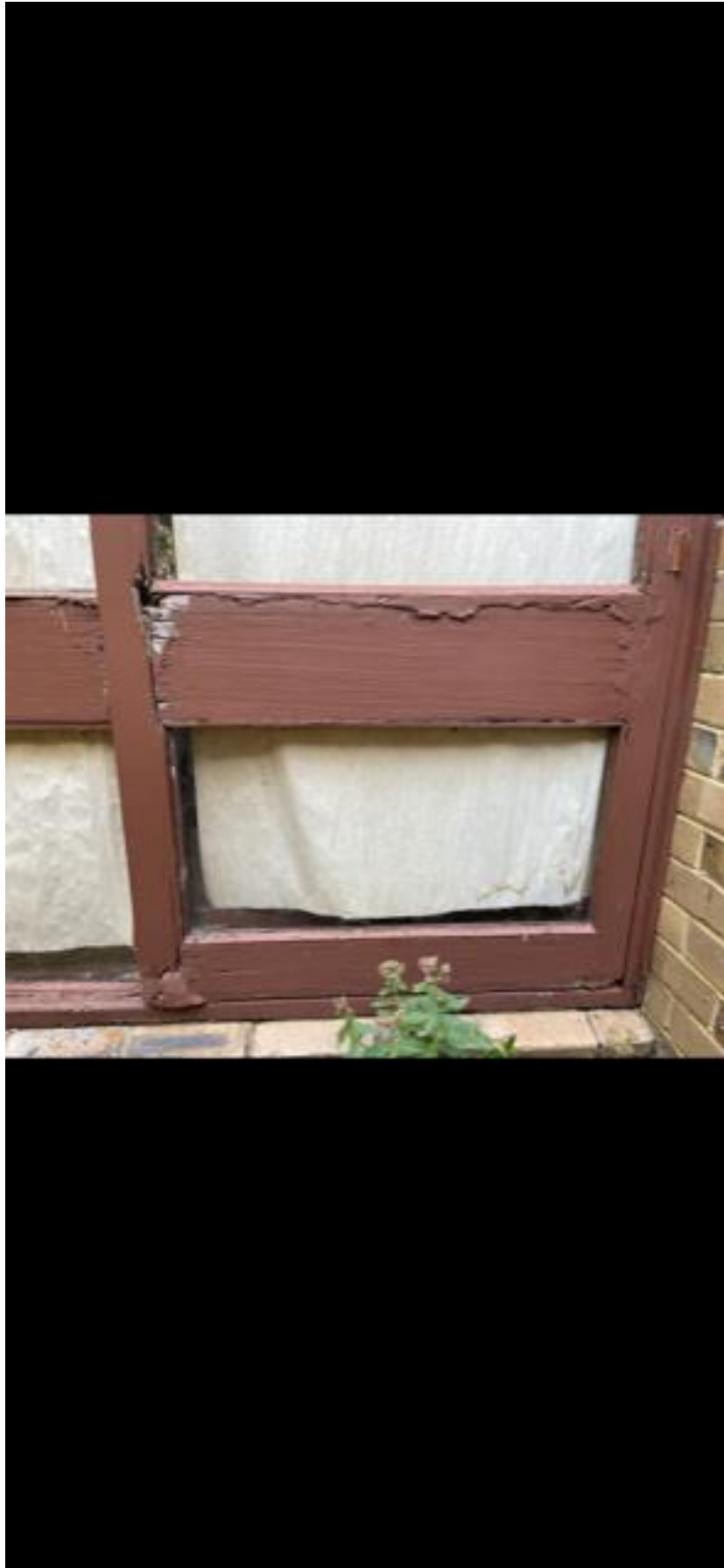
External timber cladding has deteriorated.
