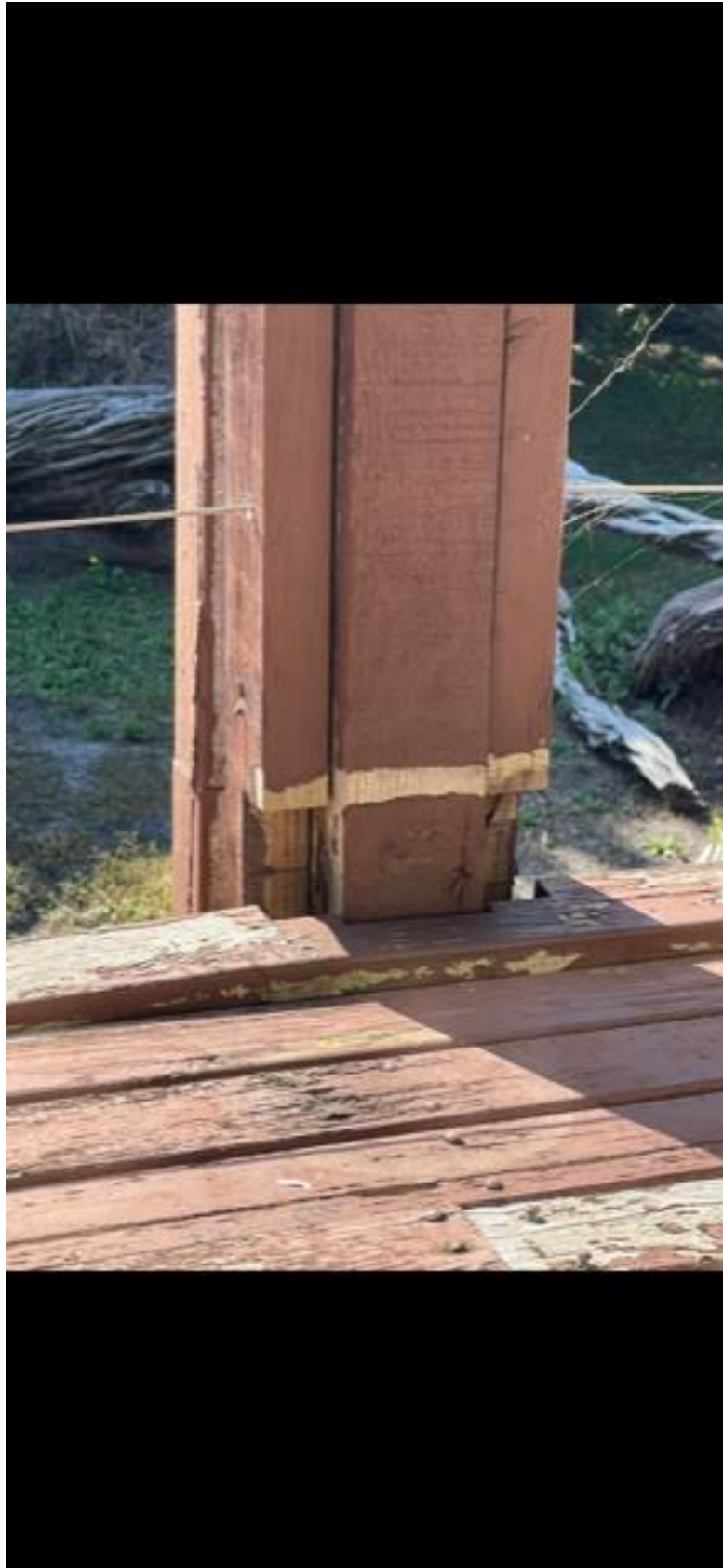
The Balcony floor has dropped
