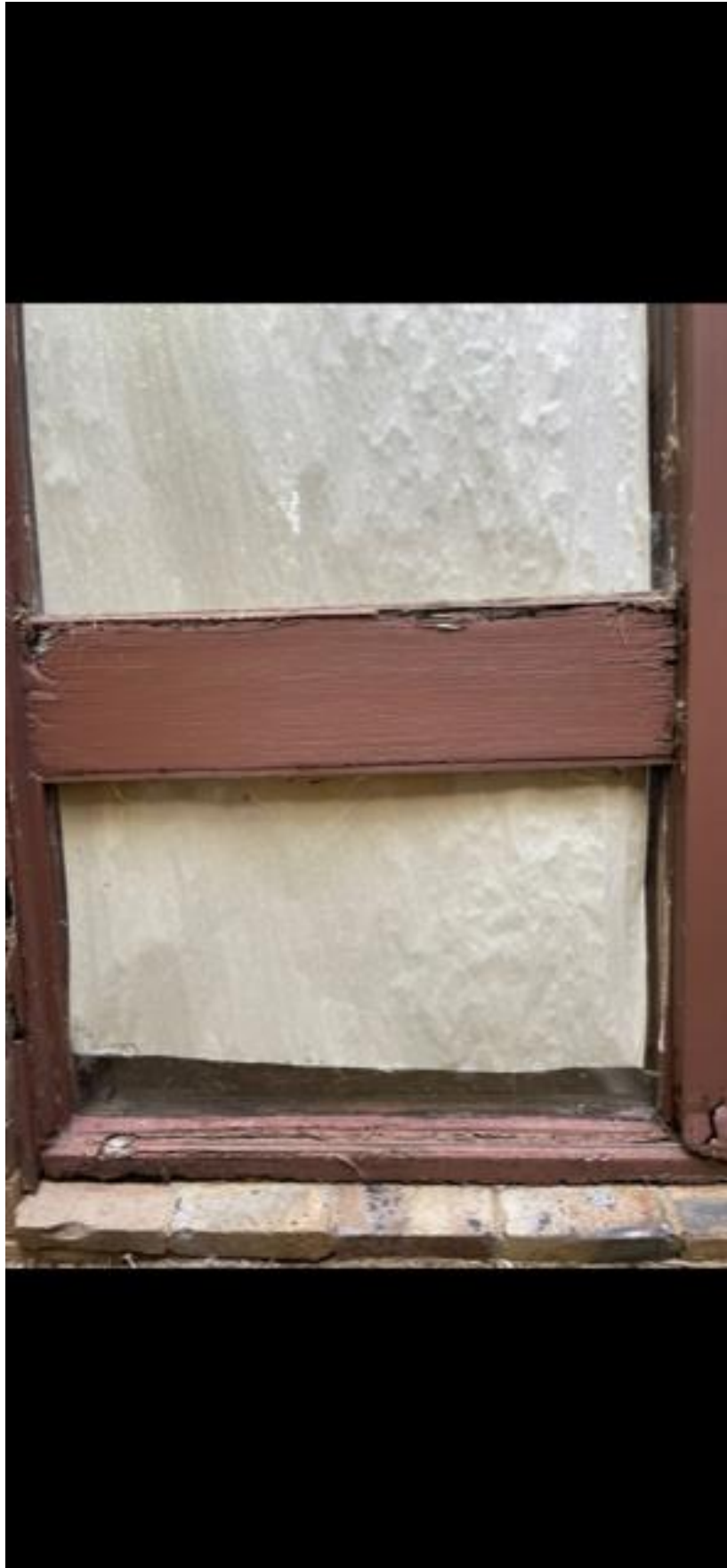
External timber cladding has deteriorated.
