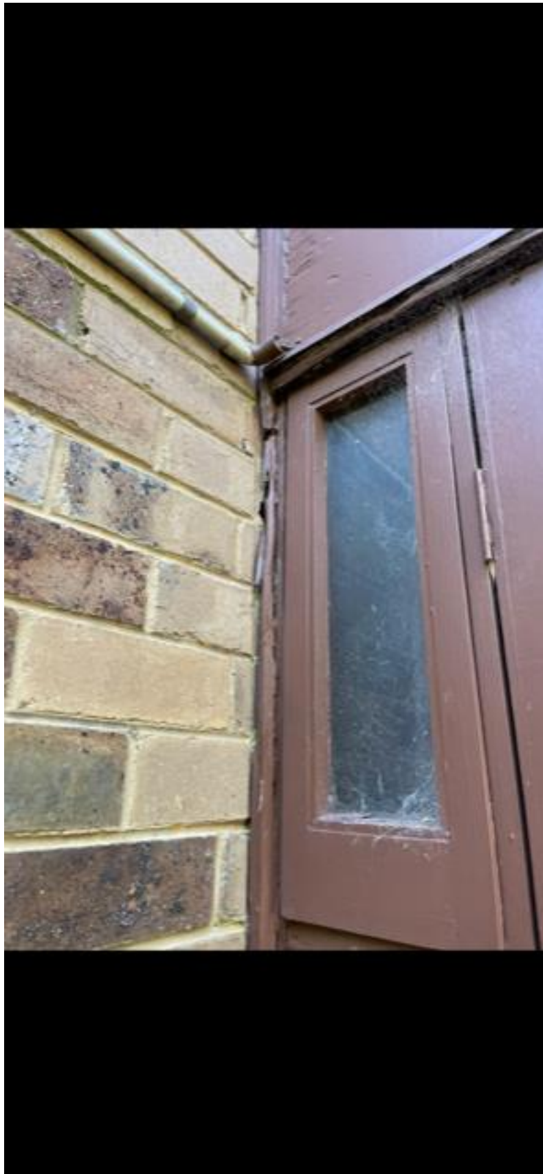
External timber cladding has deteriorated.
