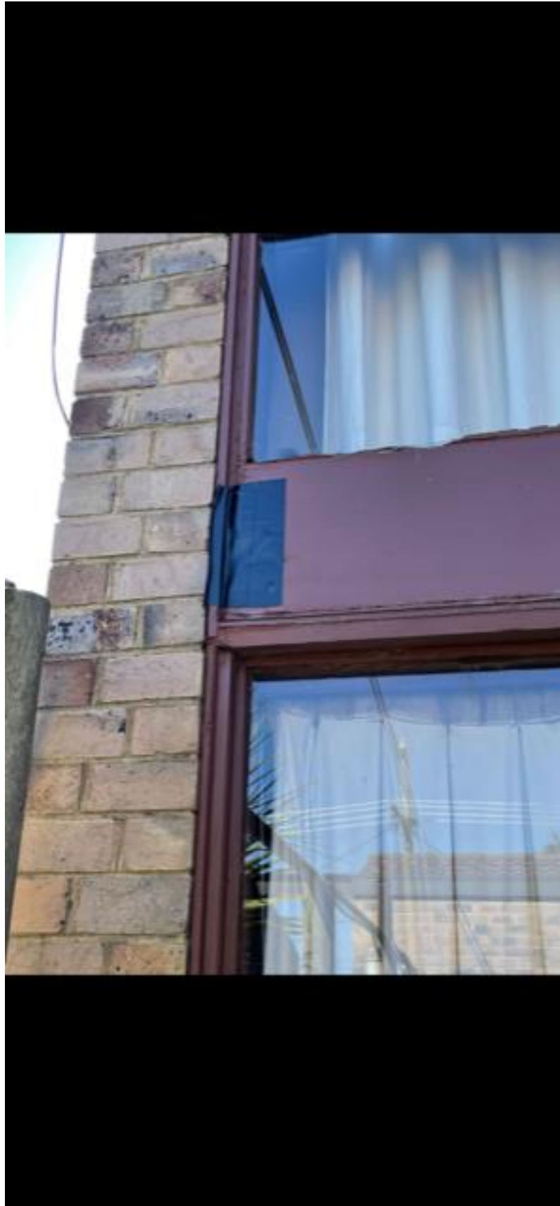
External timber cladding has deteriorated
