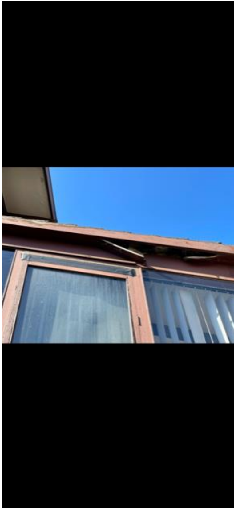
External eave lining has deteriorated
