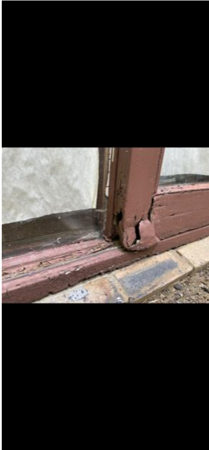
External timber cladding has deteriorated.
