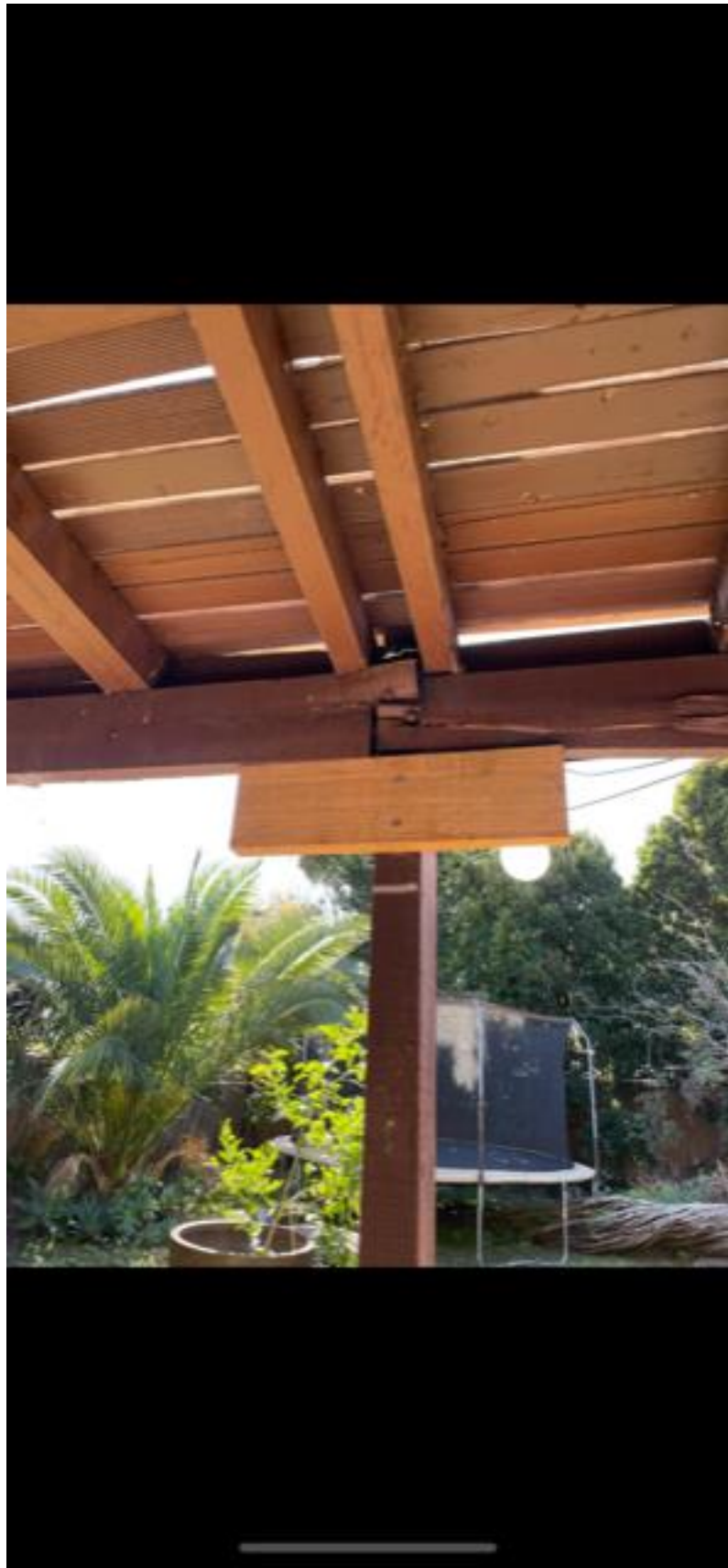
External balcony has deteriorated.
