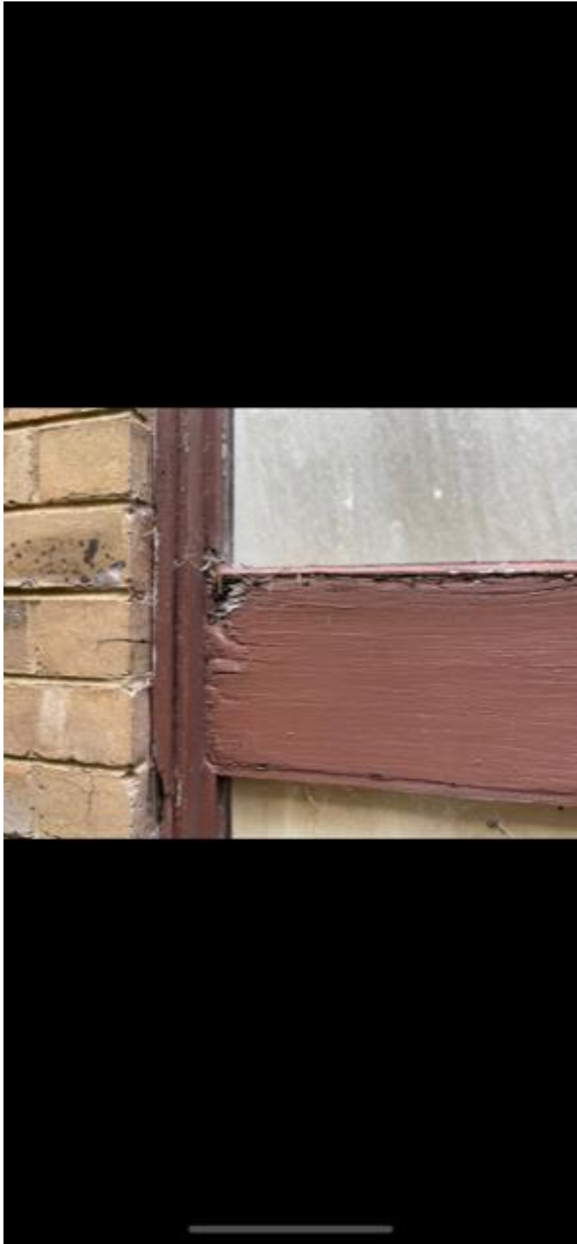
External timber cladding has deteriorated.
