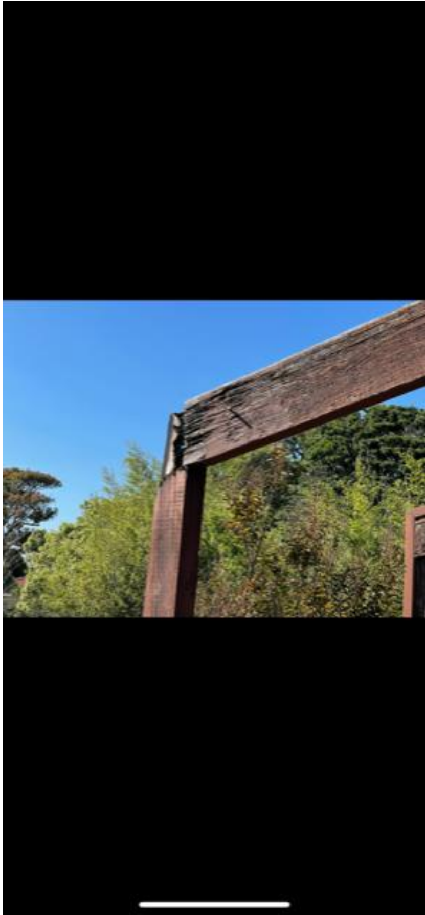
Dwelling rafters have deteriorated.
