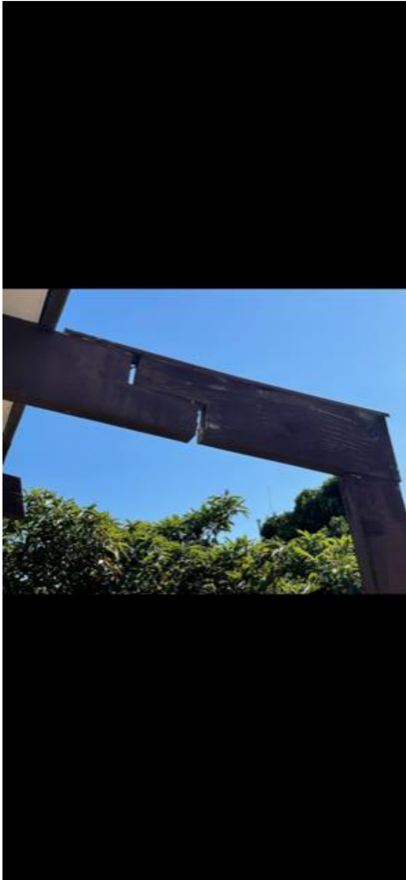
Dwelling rafters have deteriorated.
