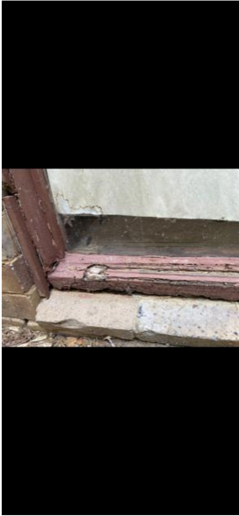
External timber cladding has deteriorated.
