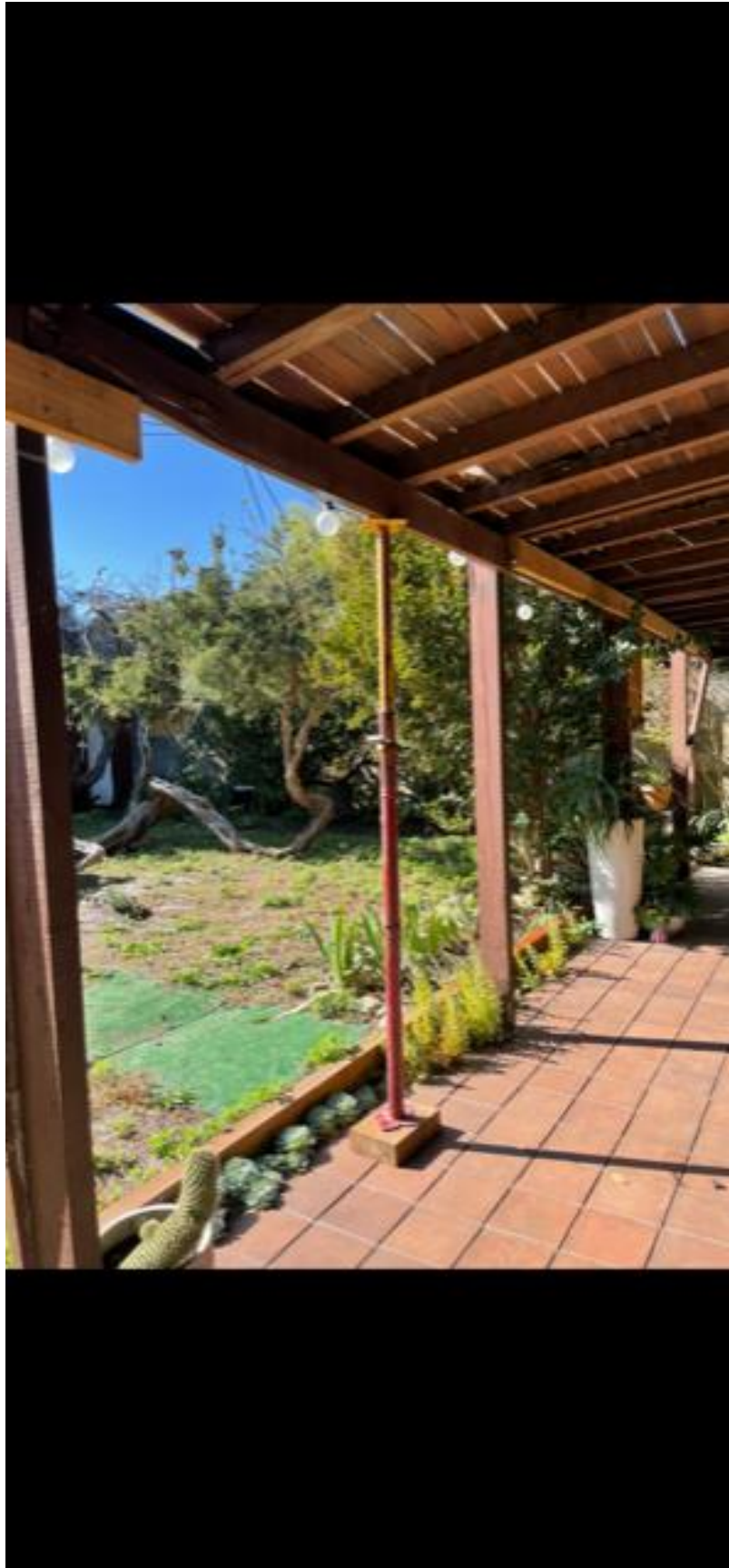
External balcony has deteriorated.
