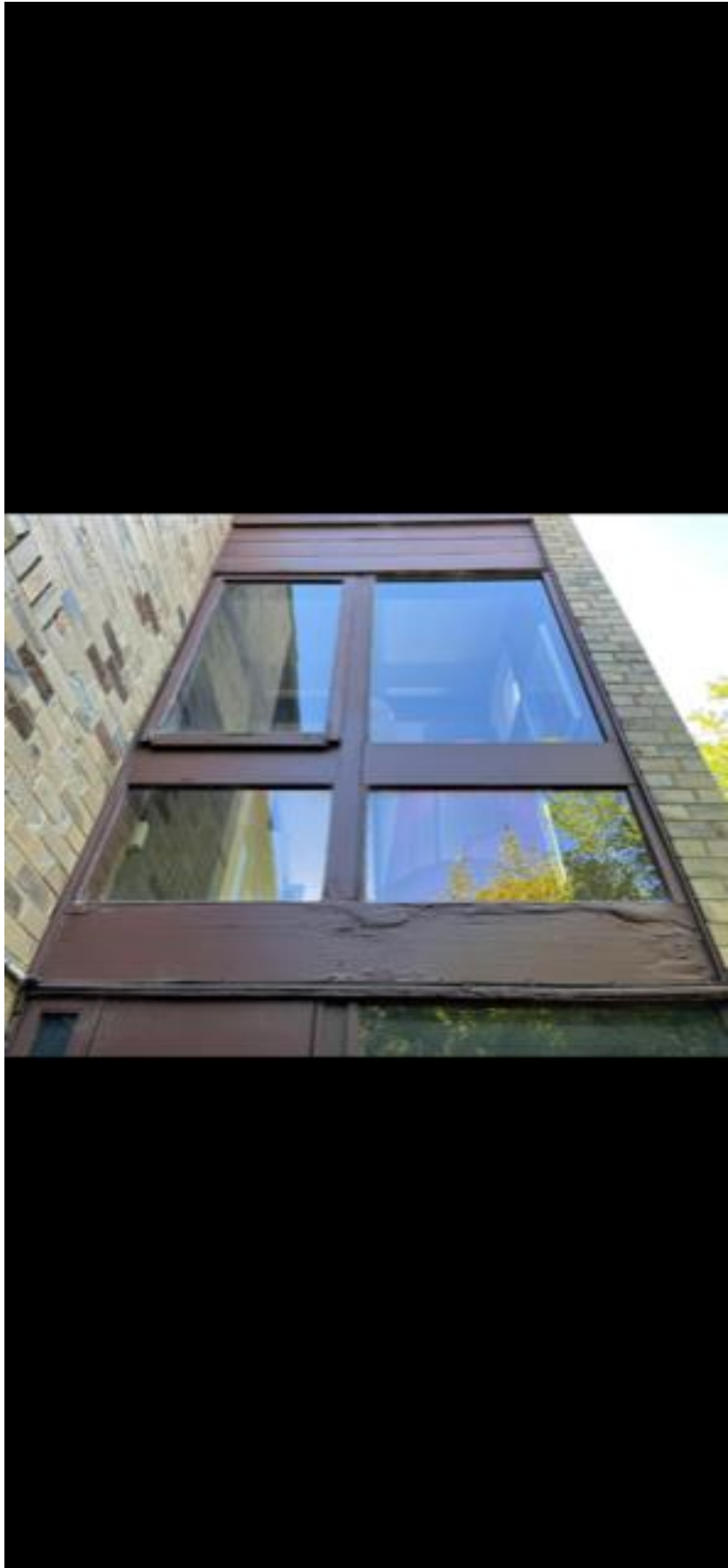
External timber cladding has deteriorated.
