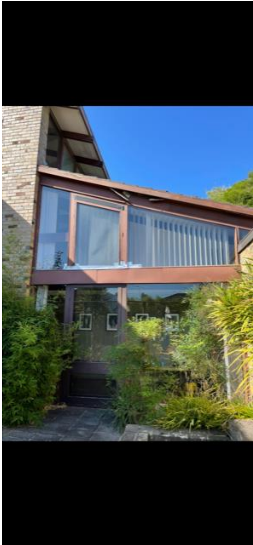
External timber cladding has deteriorated.
