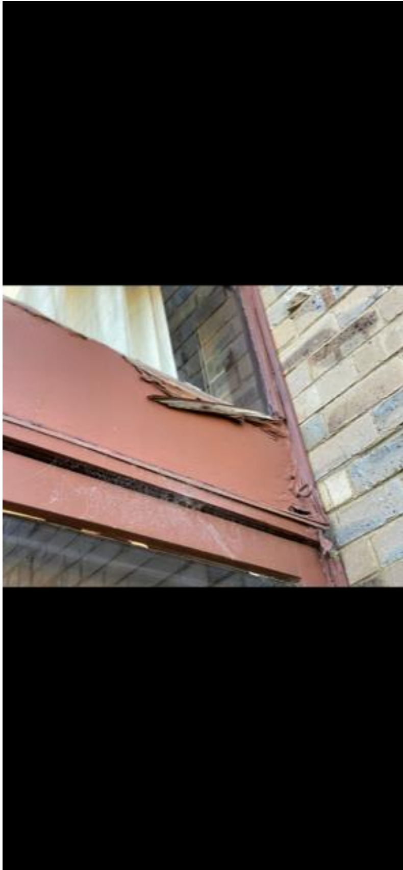
External timber cladding has deteriorated
