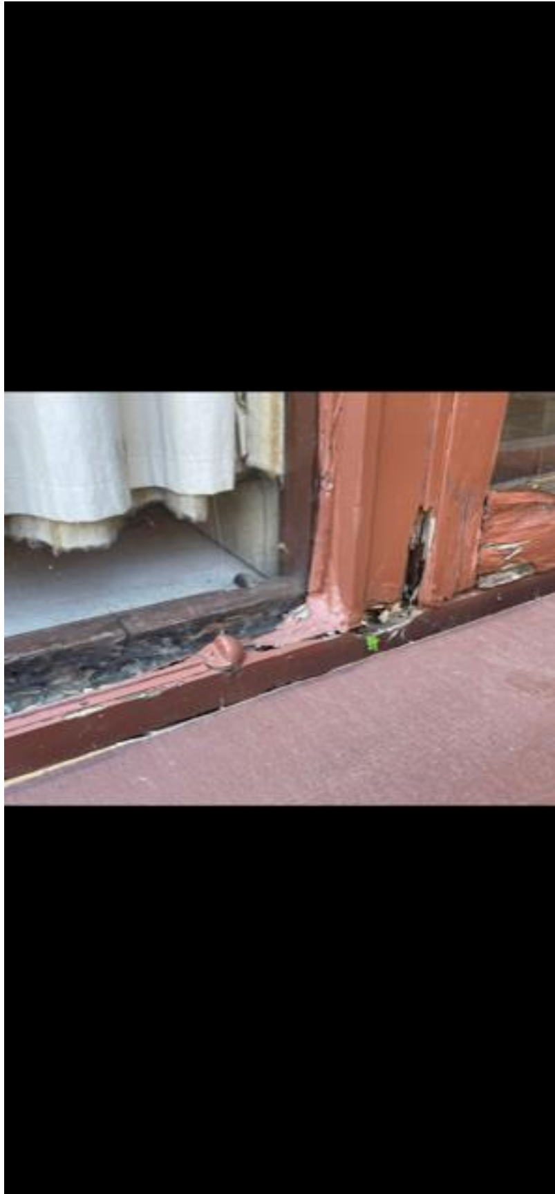
External timber cladding has deteriorated
