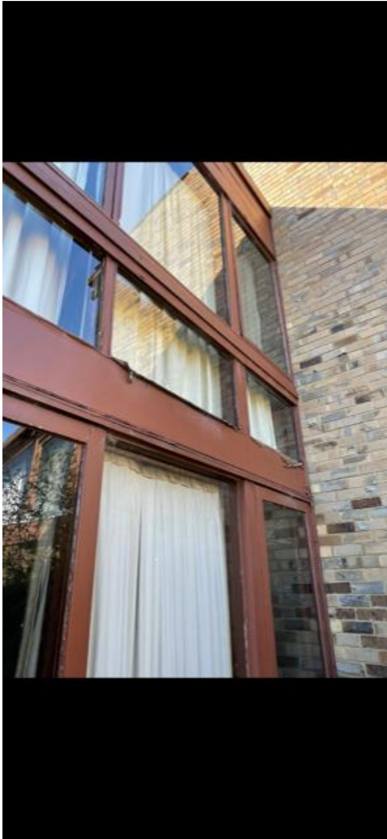
External timber cladding has deteriorated
