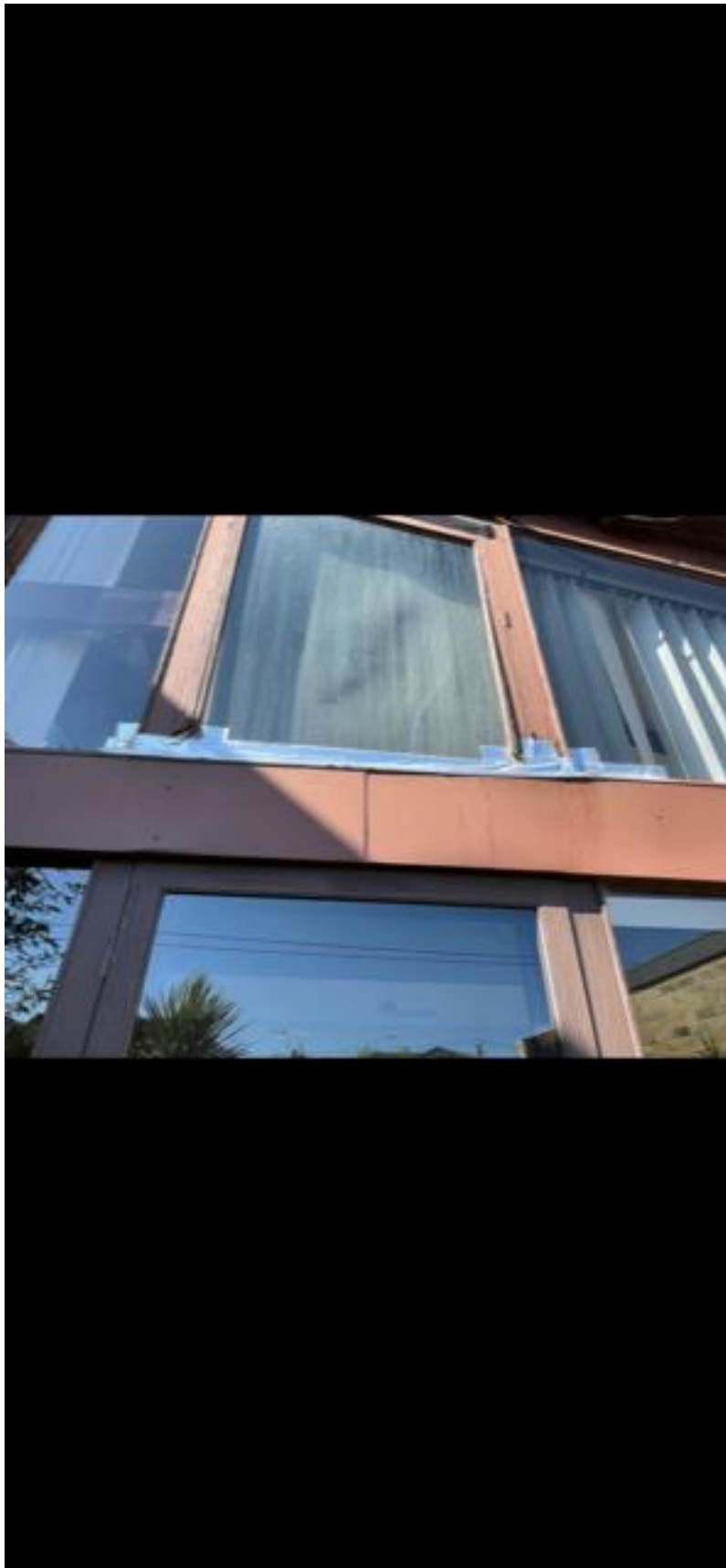
External timber cladding has deteriorated
