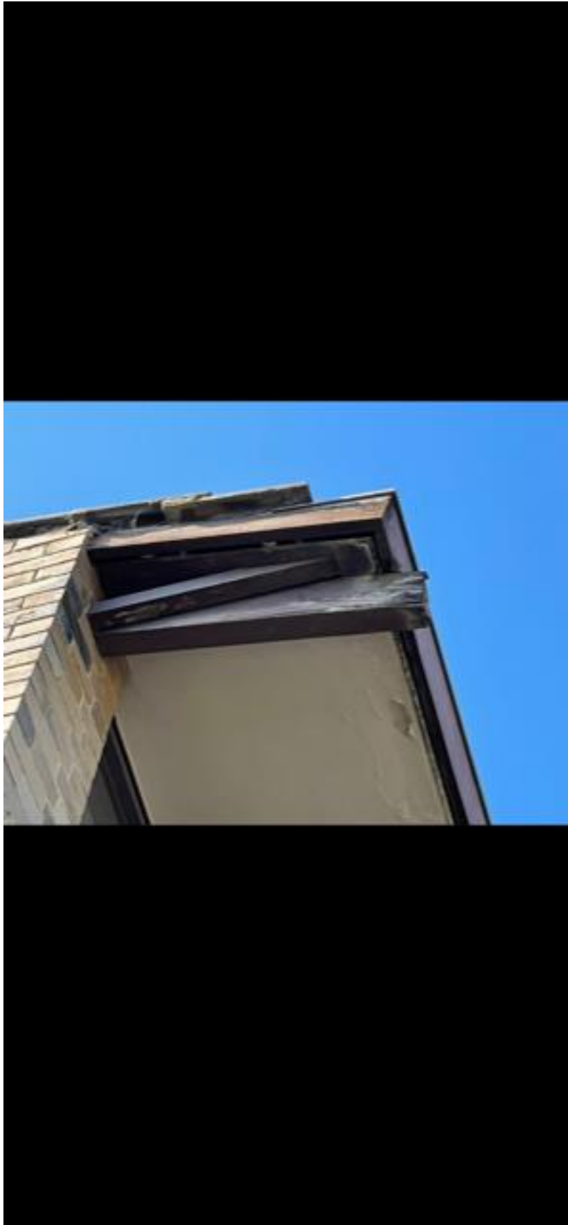
Dwelling rafters have deteriorated
