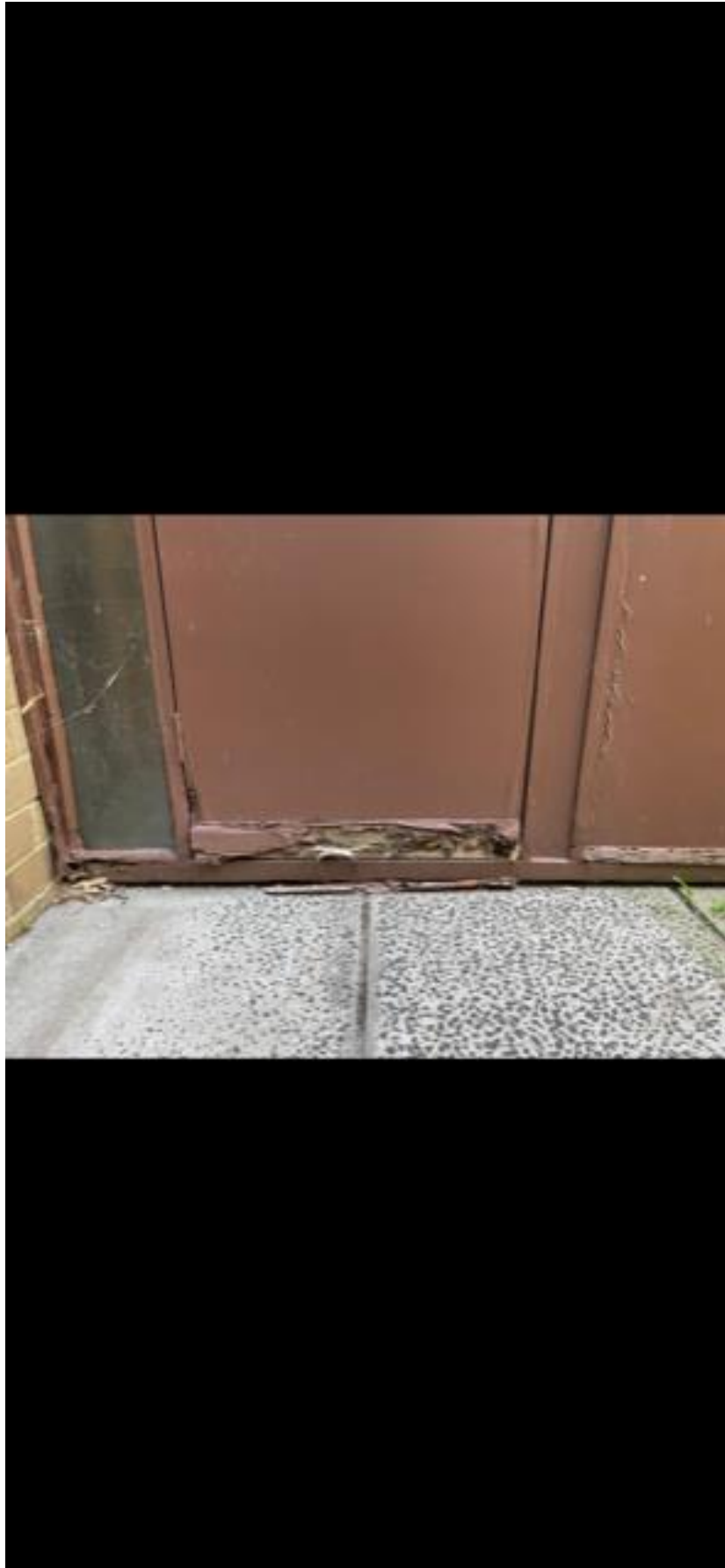
External timber cladding has deteriorated.
