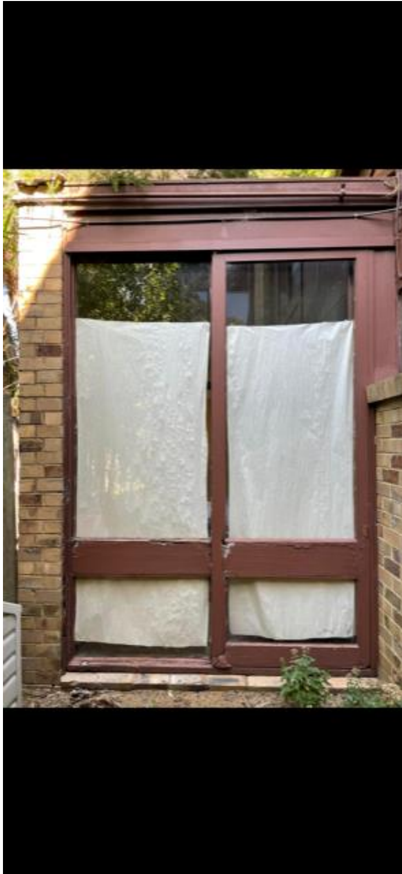
External timber cladding has deteriorated.
